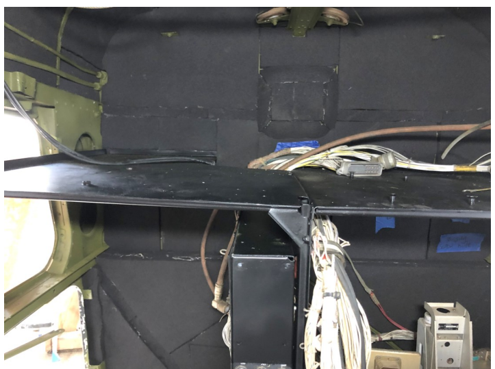
The rear radio station was a hodgepodge of military gear hiding overlapping patched panels, all of which needed attention. Top to bottom: before, during, and after the work.
